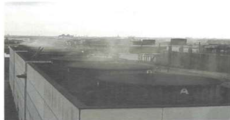
Fig. 19.1 Cooling towers—a possible source of Legionella infection.
